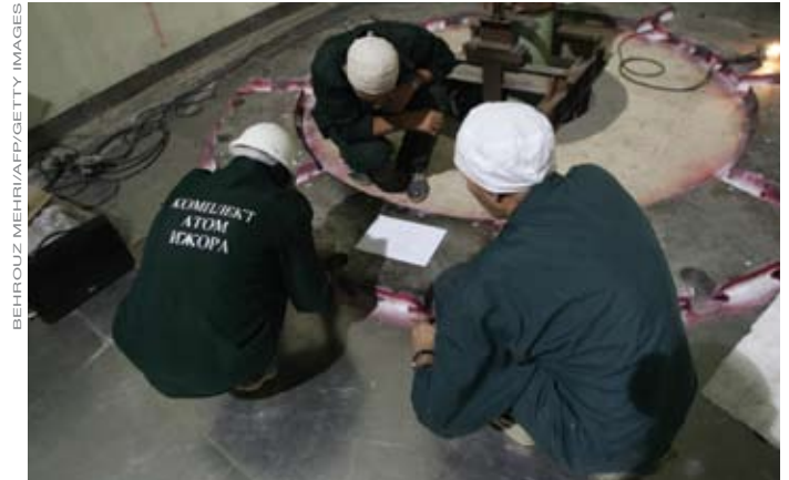
ON THE JOB Russian engineers work on a plan inside the reactor building of the Bushehr nuclear power plant in Iran.
